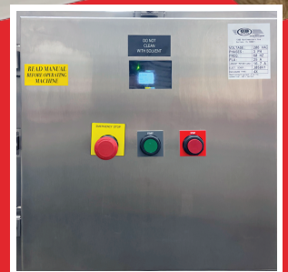
Control Panel (Opposite Side)
